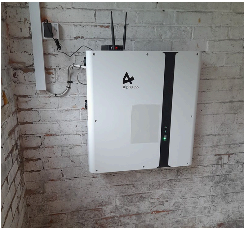
Figure 3.15 Installation of an Alpha ESS SMILE-B3 battery in an outhouse with a mobile router
