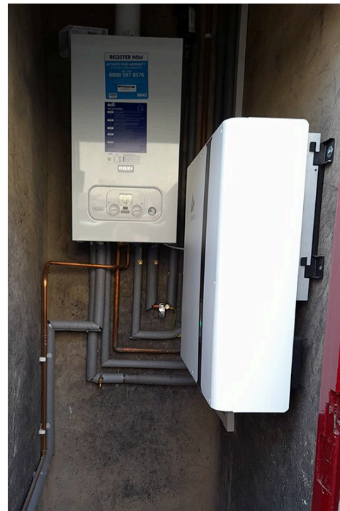
Figure 3.18 Battery installed in an outhouse with a boiler
