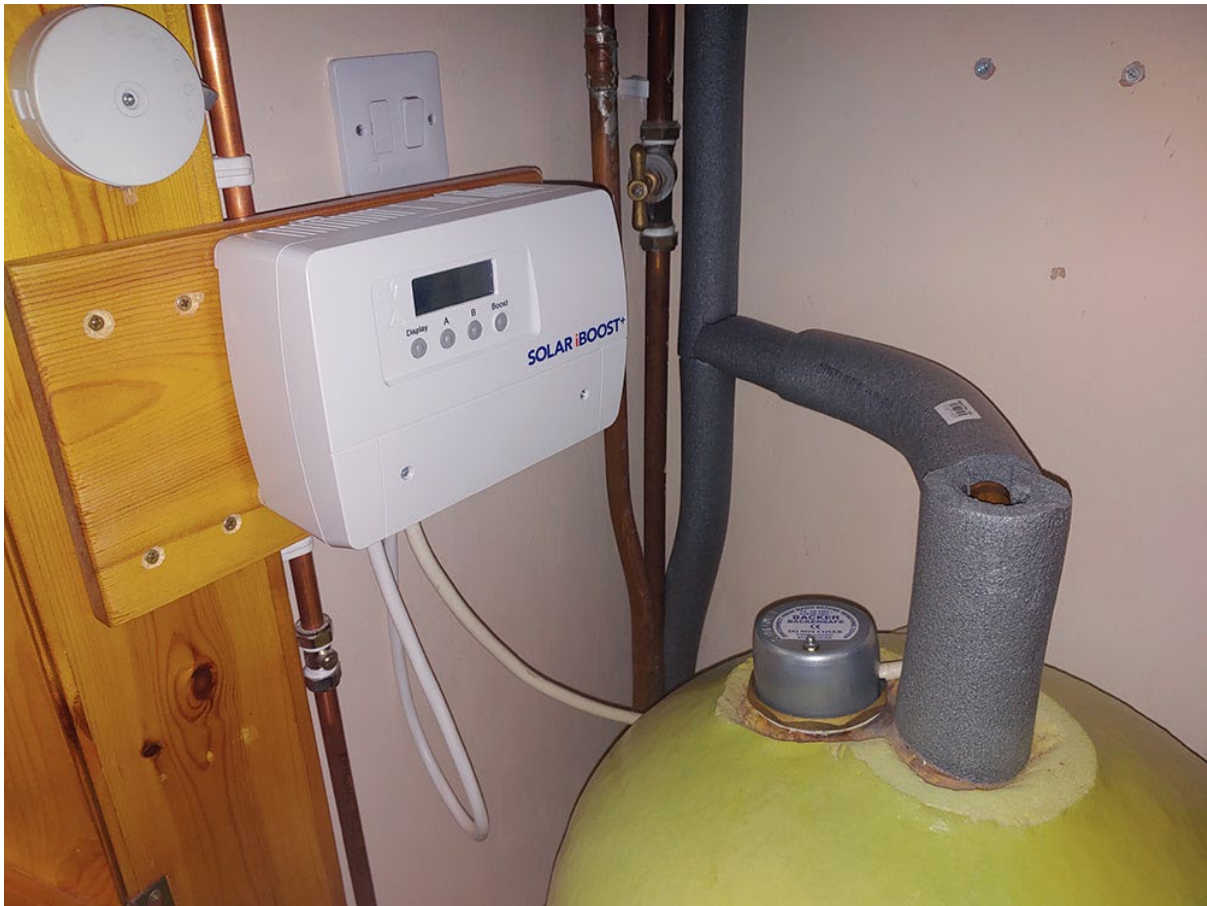
Figure 4.26 Solar iBoost+ solar immersion controller for household W-02 with the hot water cylinder and immersion heater
