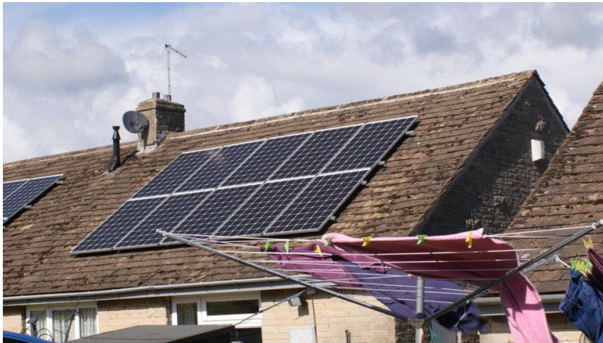
Figure 7.5 Example of Energise Barnsley solar PV installation
