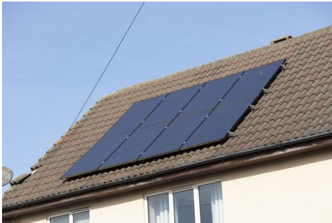
Figure 7.1 Photo of solar PV installations in Sunderland
