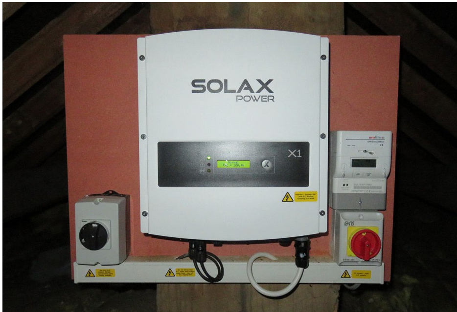
Figure 5.3 SolaX inverter with the DC isolator, AC isolator and smart generation meter
