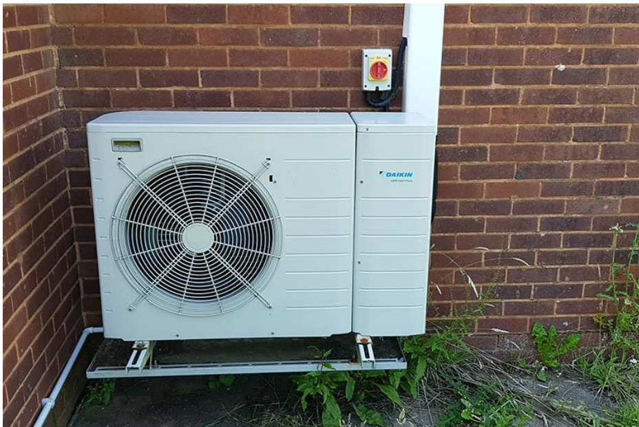
Figure 4.112 Daikin Altherma EDLQ05CAV3 air-source heat pump providing heating for household C-03
