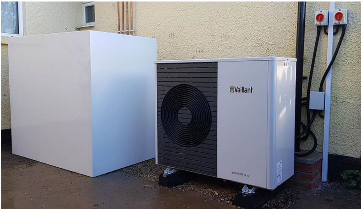
Figure 3.2 Boxergy Hero installation showing the system with the Hero Box covered
