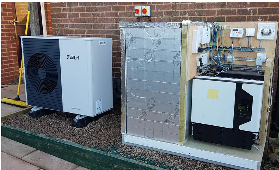
Figure 3.1 Boxergy Hero installation showing components within the Hero Box.
