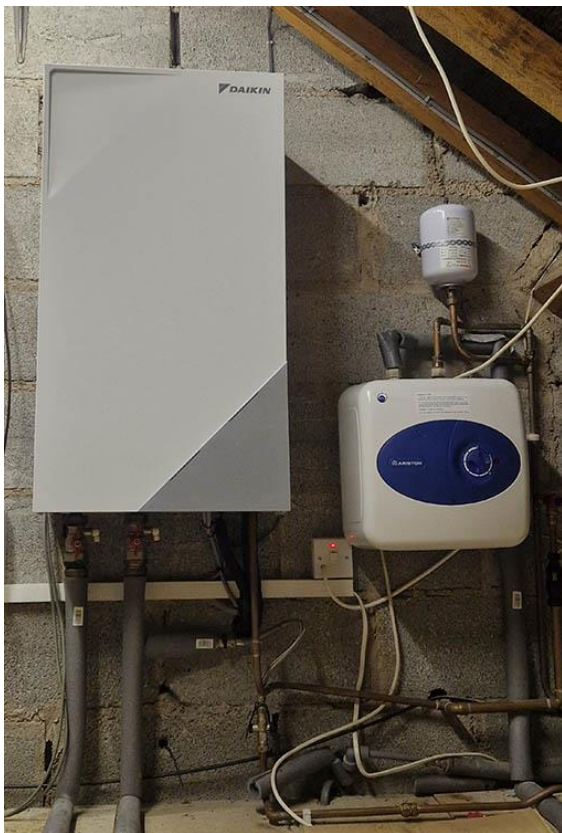
Figure 4.120 Indoor unit of heat pump and instant water heater
