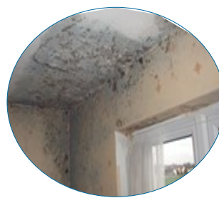
Condensation can cause mould and a musty smell
